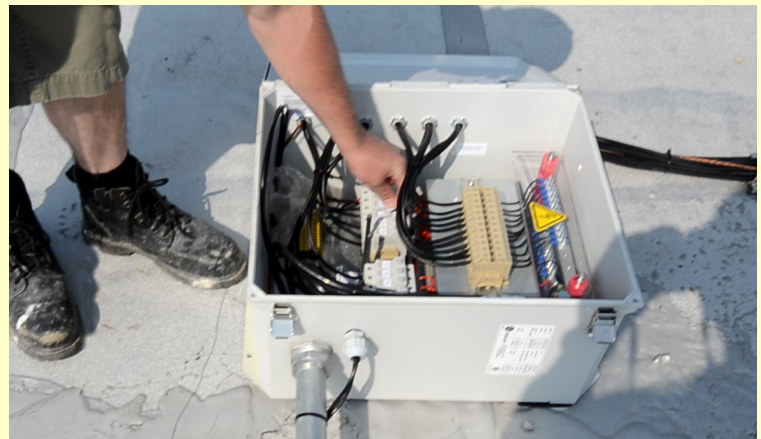
Equipment ID shows where to look for the problem
